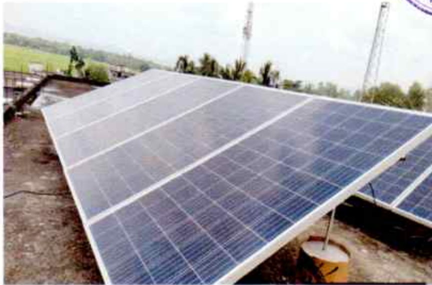
Fig 10:- Solar panels installed in Khaira College, Khaira
